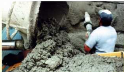
High volume shotcreting (wetgunning) with the adaptable ST-45 is all in a day's work for this versatile concrete pump.
