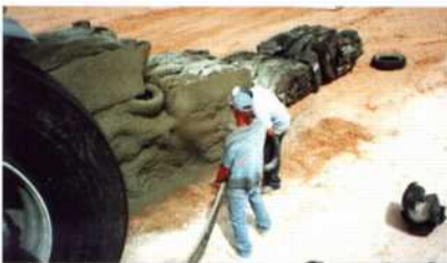
Shotcreting (wetgunning) with a stiff, low slump mix, is just one of the many uses for the ST-70 concrete pump.
